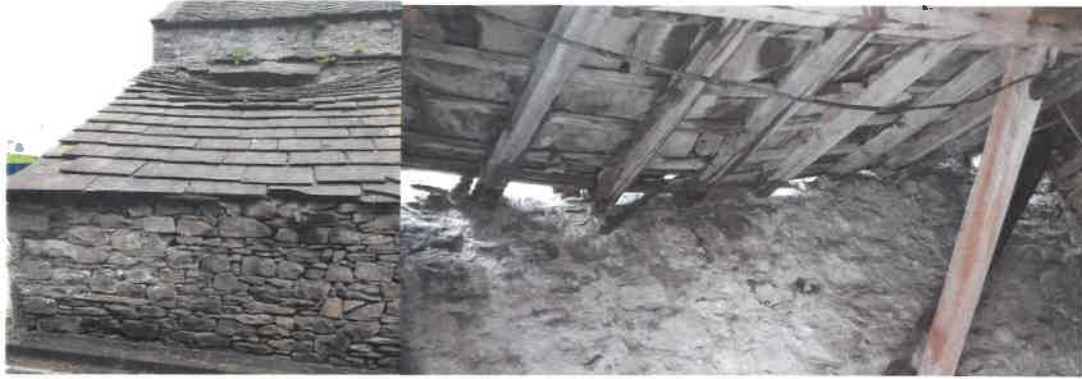
Photograph 1- Roof deterioration on the north lean -to.
