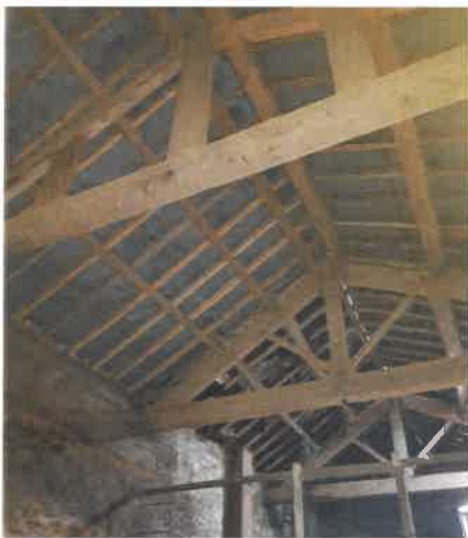
Photograph (2) – showing the good condition of the trusses purlins and rafters in the main barn.
